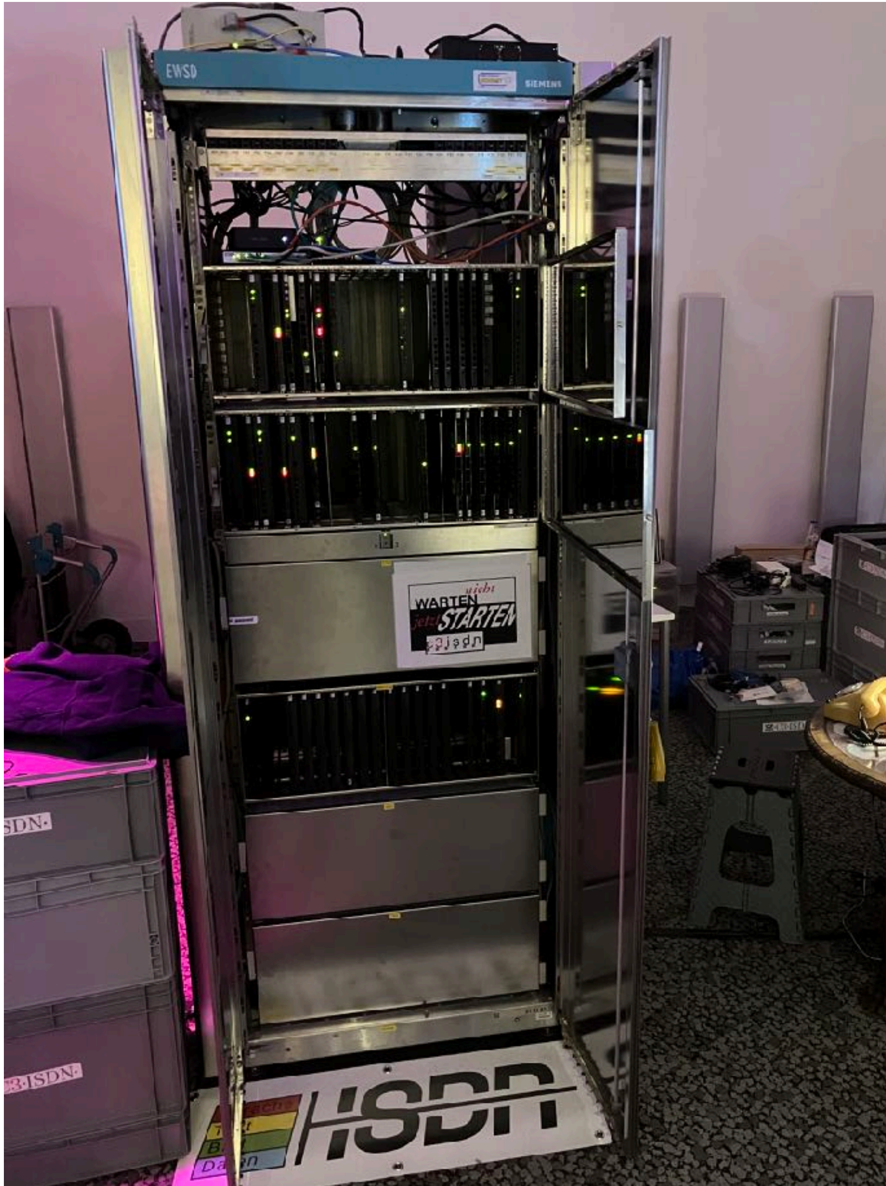
EWSD Switch installed at the 38C3
